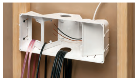
2 Pull power and low voltage wire. After installing the wall, continue with retrofit steps 3 and 4 (above).
